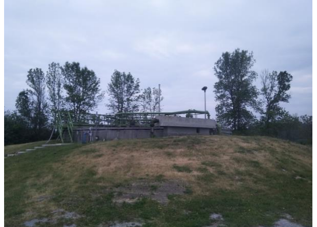
IMAGE 8 WATER TREATMENT STRUCTURE
